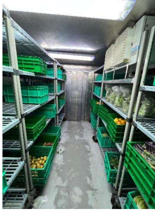
Figure 3. 20 Sofra Restaurant Walk In Chiller
