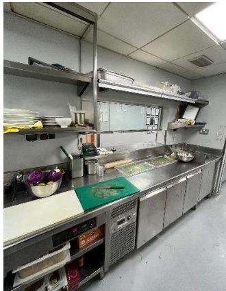
Figure 3. 13 In Room Dining Cold Kitchen
