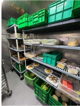
Figure 3. 22 In Room Dining Walk In Chiller
