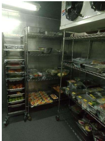
Figure 2. 8 Walk in Chiller
