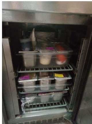
Figure 2. 6 Under Counter Chiller
