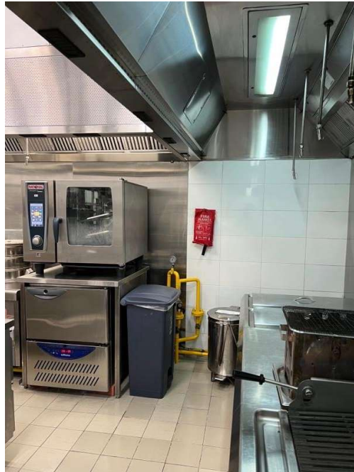
Figure 3. 13 Grill and Oven Area
