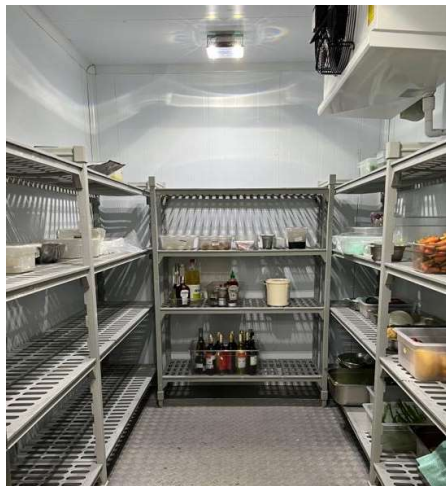
Figure 3. 11 Pink Pearl Standing Chiller
