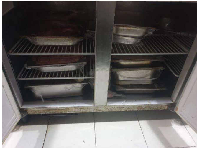
Figures 3.15 Chamas Kitchen Cold Kitchen Chiller
