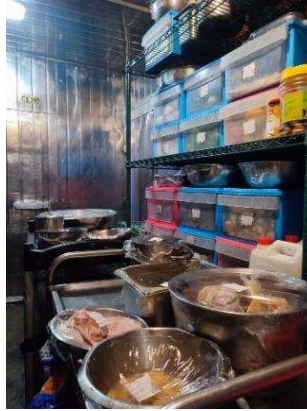
Tang Palace Chiller
