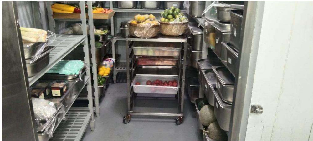
Figure 2. 5 Cold Kitchen Chiller
