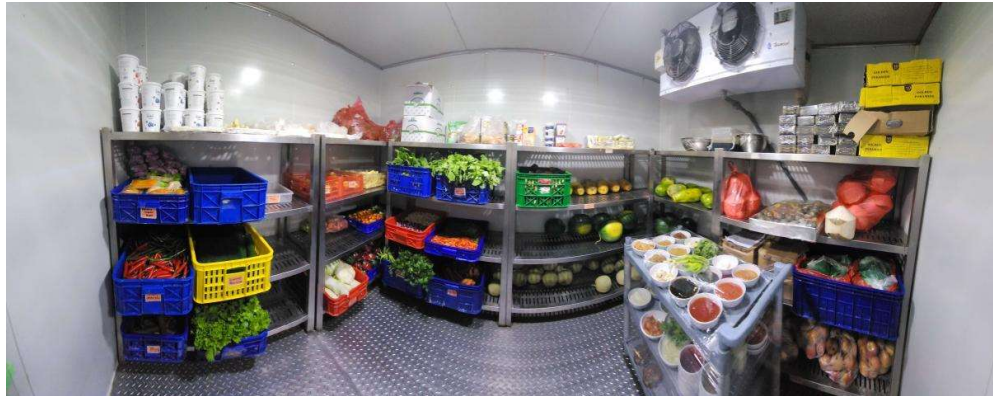
Figure 3. 13 Walk in Chiller
