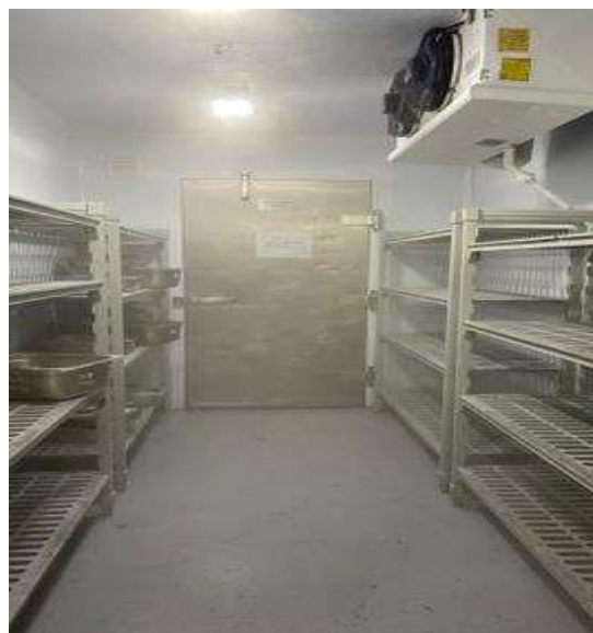
Figure 2. 7. Deep cleaning walking chiller
