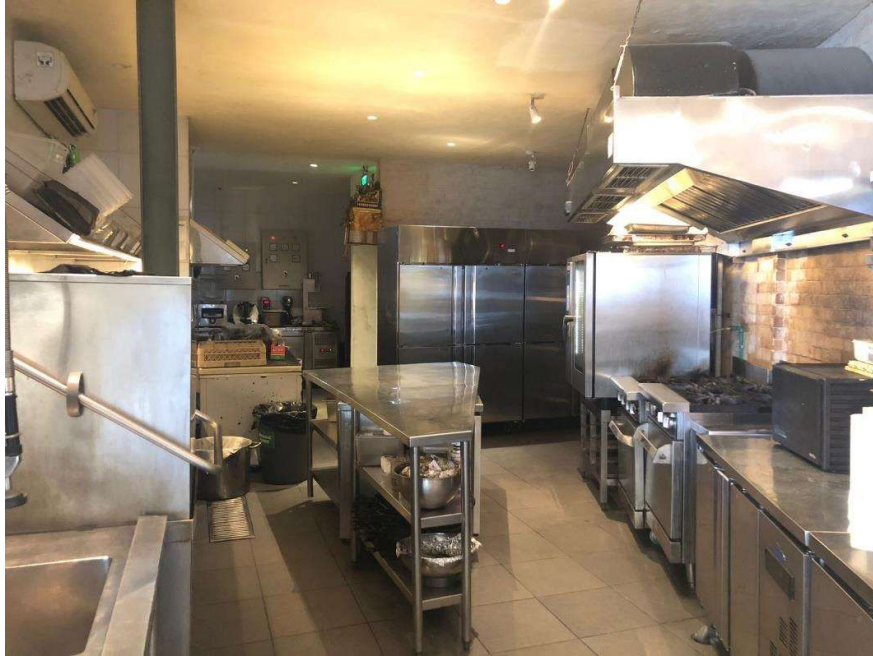
Figure 3.10. Preperation Area ( for preparation and washing )
