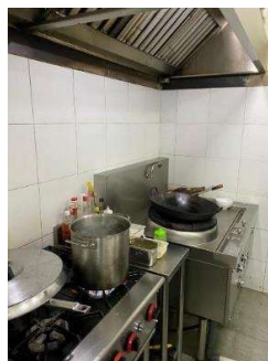
Figure 3. 29 Work & Burner Station
