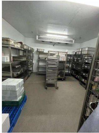
Figure 3. 42 Inside General Freezer
