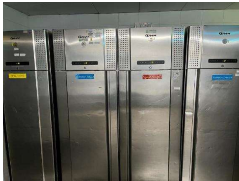
Figure 3. 18 Chiller and Freezer
