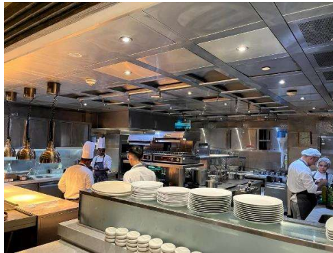
Figure 3. 45 Rockfish Service Kitchen
