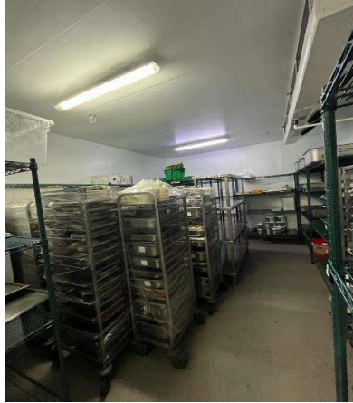
Figure 3. 40 Inside Palmery Chiller
