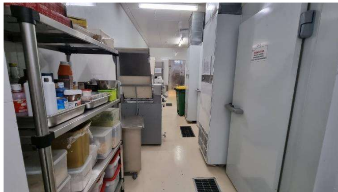
Figure 3. 20 Chiller and Freezer
