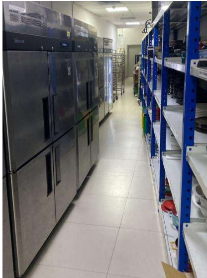
Figure 3. 35 Chiller and Freezer Corridor
