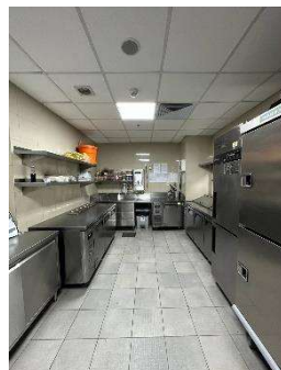
Figure 3. 45 GDM Section Kitchen
