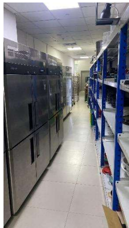
Figure 3. 49 Chiller and Freezer Corridor
