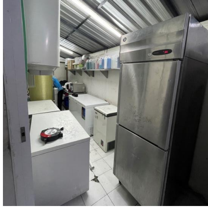
Figure 3.37. Chiller and Freezer
