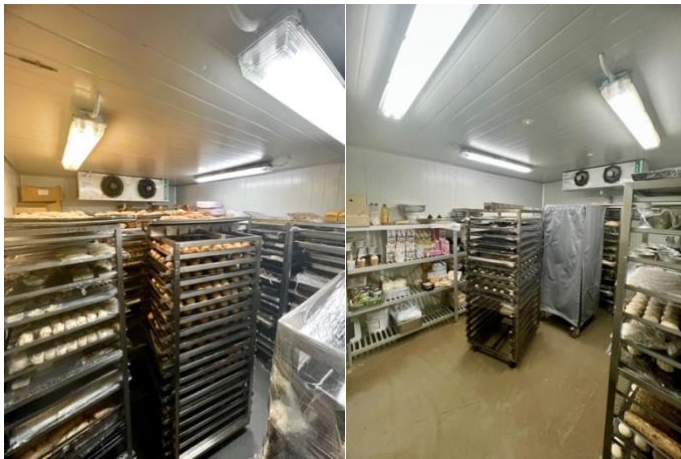
Figure 37. Freezer & Chiller Pastry Kitchen
