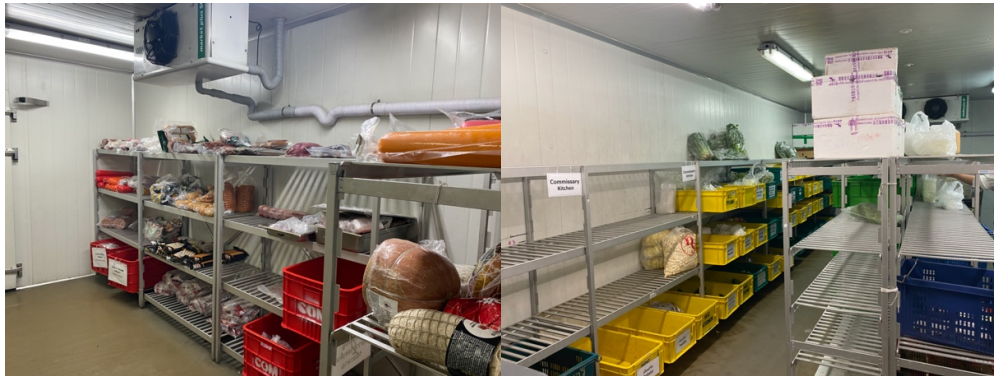
Figure 3.17 Walk In Chiller
