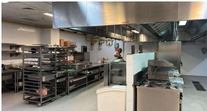
Picture 21 Renaissance Main kitchen
