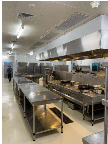
Picture 18. Hot Kitchen
