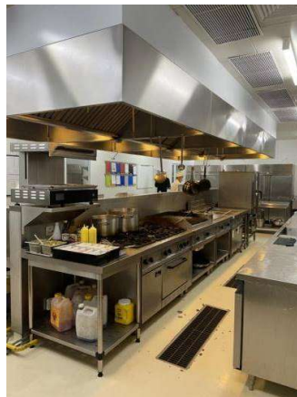
Picture 17. Hot Kitchen
