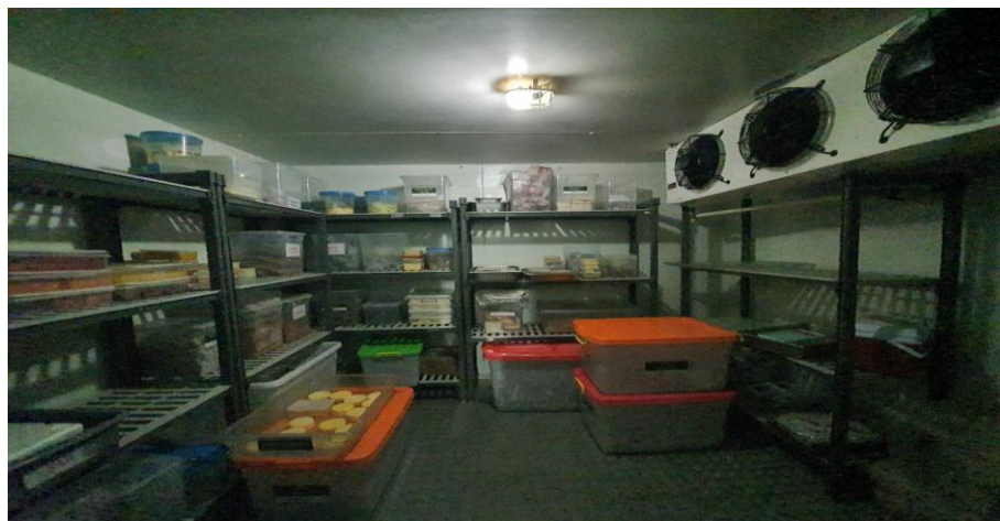
Picture 15. Walk-In Freezer (Personal Documentation, 2021)
