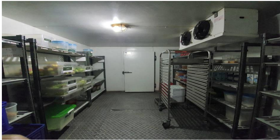
Picture 14. Walk-In Chiller (Personal Documentation, 2021)
